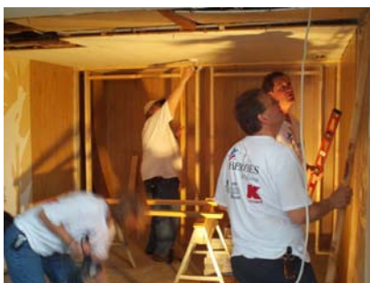
The Sears Heroes At Home Project gets an entirely new basement bedroom addition.
