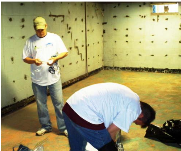
Mike Mantai and Don Clark work hard on the Lowe's Project basement
