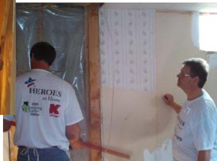
Board member Jim Banning looks on as the new walls are going in.
