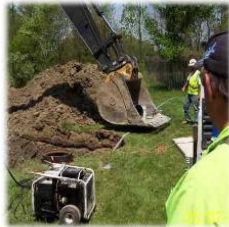
Town Utility Operator Larry Melvin checks on the sewer line work on the new detention pond that is going in behind the Community Center. Here, the contractors are tapping in the new 8" Sewer Line that will clear the way for the pond to go in.
